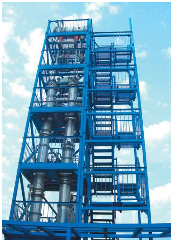
Fig. 2. Column equipment equipped with "Chevron" series mesh nozzles (JSC "Elektrogorsk Institute of Oil Refining")
