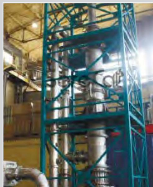
VOC emission disposal unit for SIBUR-Khimprom JSC
