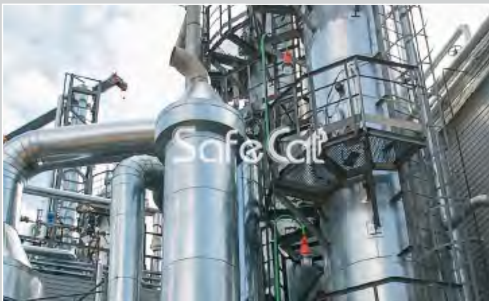
Gas treatment system of ST IG as part of a plant for the production of UFC and low methanol 55% formalin
