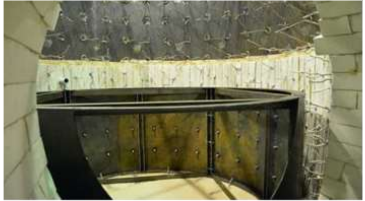
FIG. 2. Lining operations of a tube furnace at the production site of ST IG
