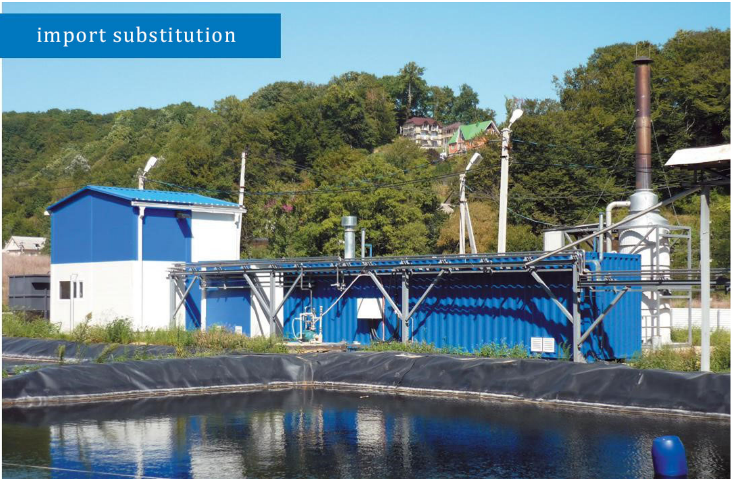
Leachate purification system (LPS) of MSW landfill, Adler
